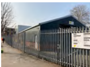
STEEL PALISADE FENCING
